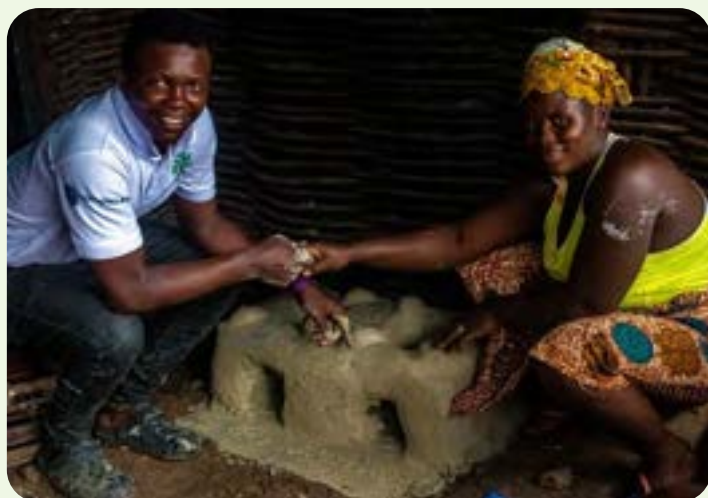
Efficient cookstove newly installed in community member's home © T.J. Blade @ Envizage Concepts
